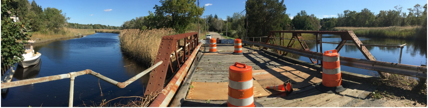
Marshallville Bridge , a "Pony Truss " bridge on Marshallville Road over Mill Creek, in the Tuckahoe Historic District, Cape May Co.
